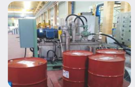
FLUSHING OIL FILLING
