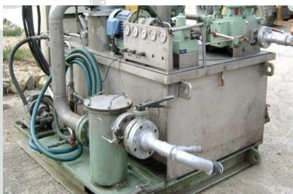
Oil Flushing Unit
