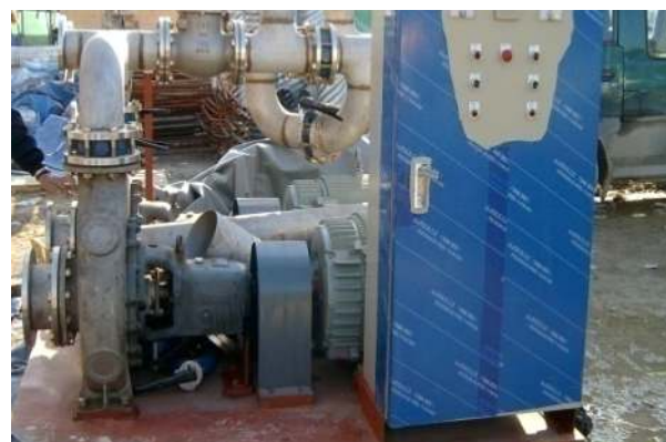
Circulation Pump Unit
