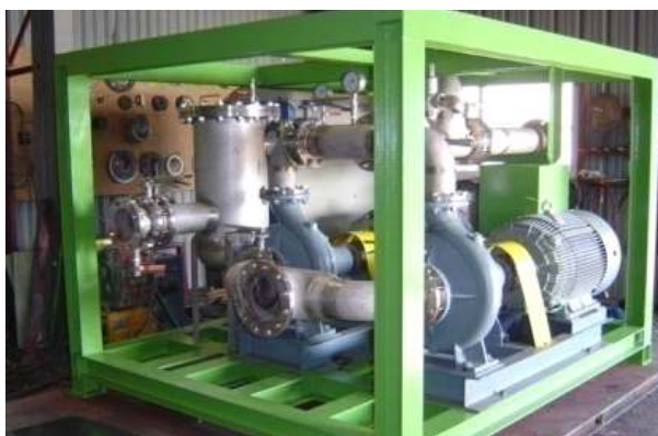
Circulation Pump Unit
