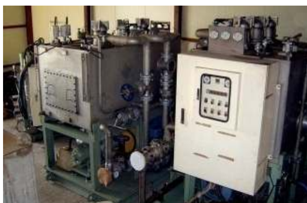
Oil Flushing Unit
