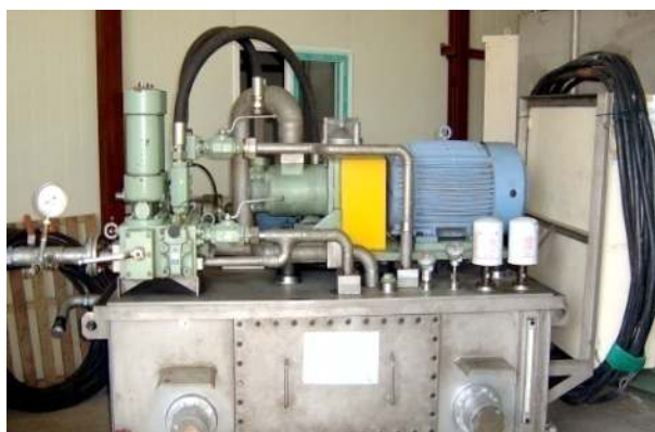
Oil Flushing Unit
